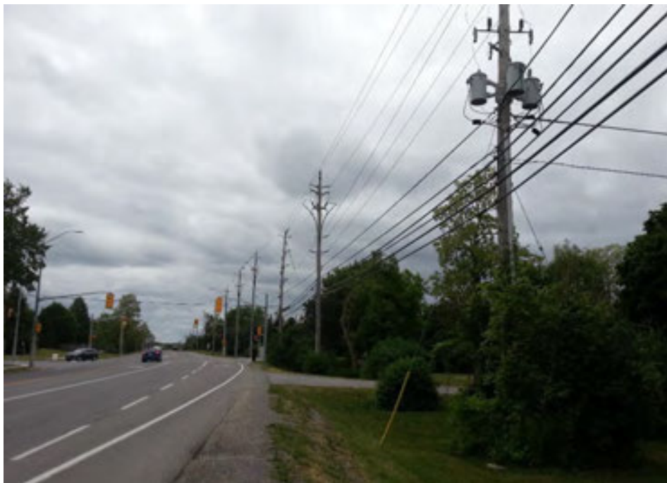
Photo 18: Looking south down Kingston Road 15 at the intersection with Gore Road. Pole mounted transformers are visible in the top right of the photograph.
